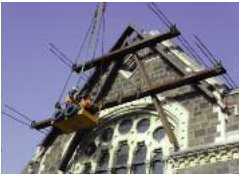
Strand and bar tendons installed through temporary structural steel frames at gable wall ends must hold the Great Hall together until a permanent repair solution can be found.
