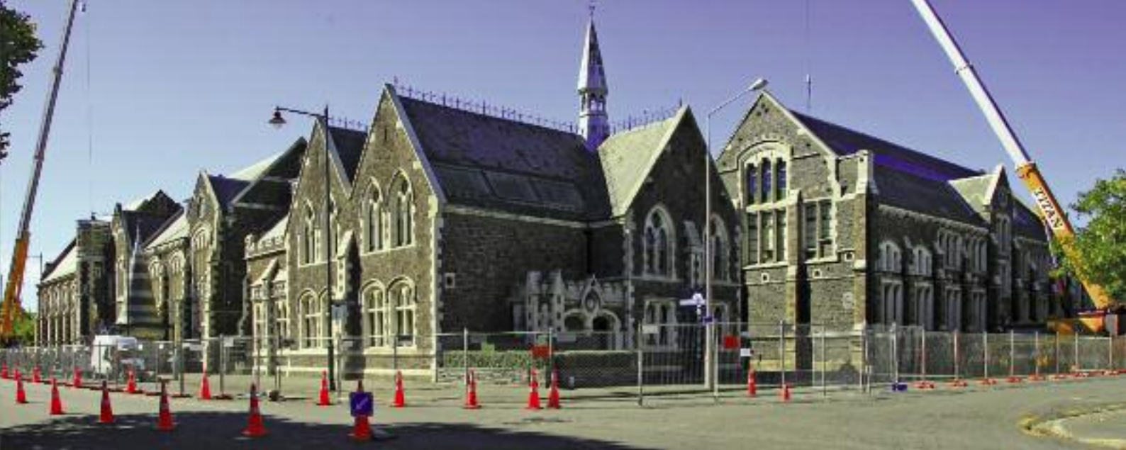
Strengthening work carried out earlier by BBR Contech contributed to the resilience of Christchurch Arts Centre's Old Arts School.
