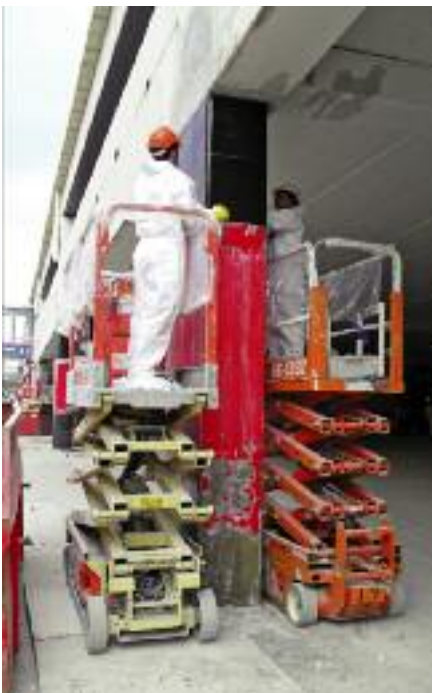
BBR Contech carried out concrete repairs at The Palms retail centre after the February earthquake.
