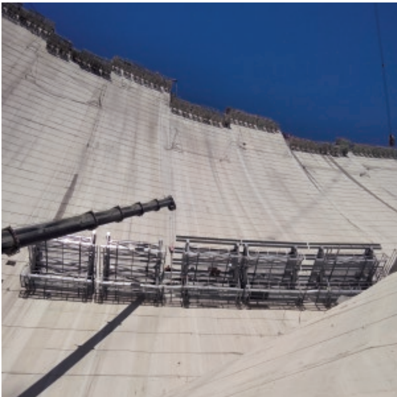
The design of the steel sluiceway bridge, which is being installed using BBR H500 Bars, for the Yusufeli Dam in Turkey allowed the contractor to fabricate the access road without interrupting the construction of the main dam wall.
