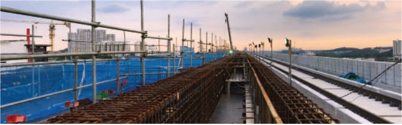
BBR Malaysia proposed an alternative post-tensioning installation solution for the two beams being constructed for the overhead Taman Putra Permai Station on the Line 2 of the Klang Valley MRT Project.
