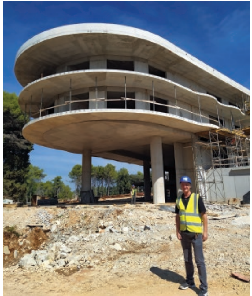
At the Hotel Pical site, BBR Adria's project manager Predrag Presečki and team-mate Dejan Buha in the background stand beside the hotel's newest architectural feature – only achievable with BBR post-tensioning technology and expertise.
