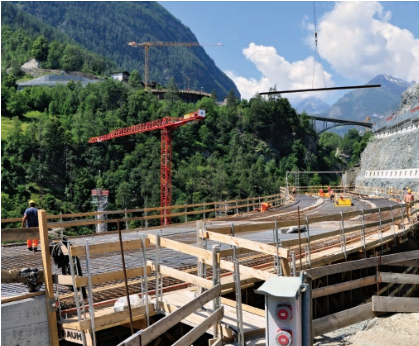
With a deck realized using BBR VT CONA CMI internal tendons, the 270m-long Chinegga Bridge stretches in a wide bend, some 60m above the Mattervispa Valley.
