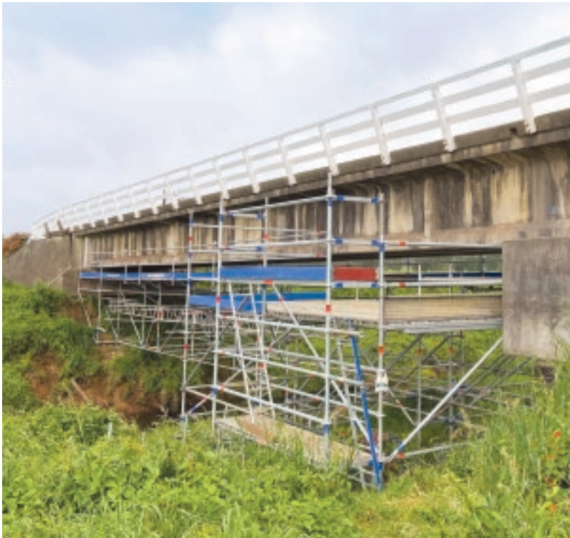
Waihue Bridge, north of Dargaville in Northland's Kaipara district of New Zealand, is one of several such structures originally built in the 1960s to 1970s and which now needs strengthening.
