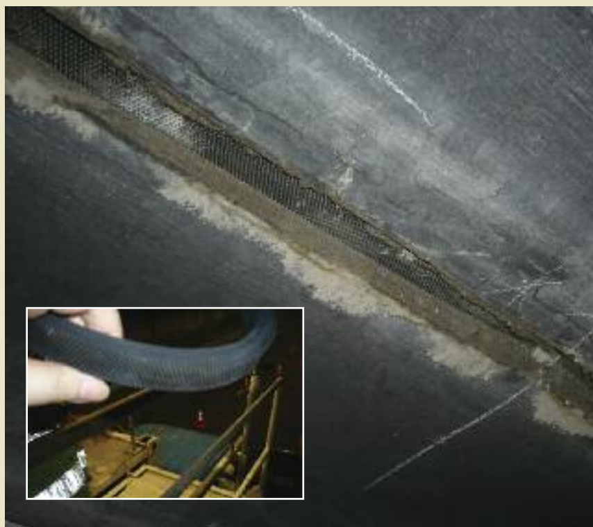
CATHODIC PROTECTION, CENTRAL EXPRESSWAY, SINGAPORE
