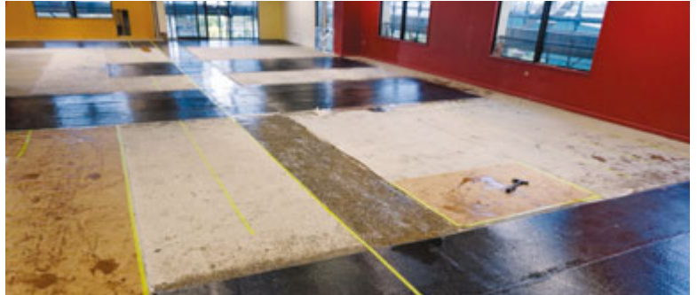
Strengthening work and repairs to the floors were carried out by BBR Contech at the Allied Telesis Labs New Zealand campus in Christchurch.
