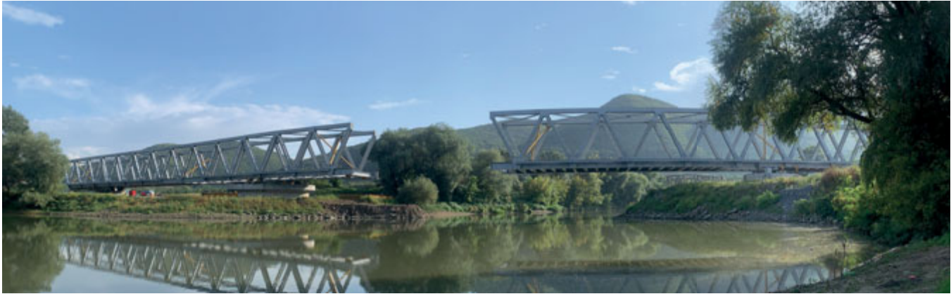
Before connecting the two bridge sections, they were aligned longitudinally and transversally using hydraulic jacks.
