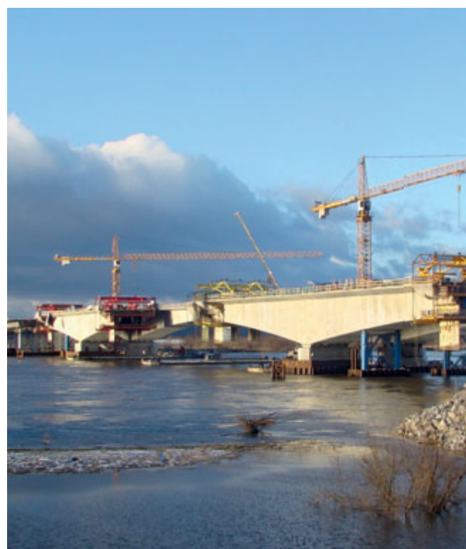
2011 – Grudziadz Bridge, a milestone in cantilever construction, pictured here just before span closure took place.
