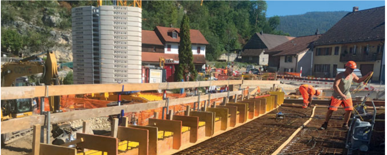
The new Recolaine Bridge features CONA CMI EIT post-tensioning which offers the highest corrosion protection level for maximum durability.
