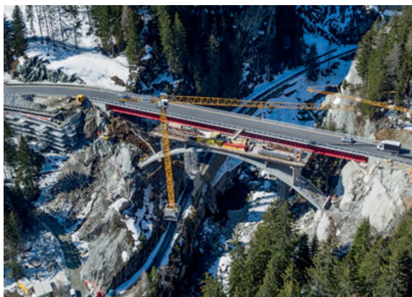
Aerial view of reconstruction work underway for the Crestawald arch bridge. The adjacent temporary bridge carries traffic on the A13 National Road during the works. Image courtesy of Bundesamt für Strassen ASTRA.
