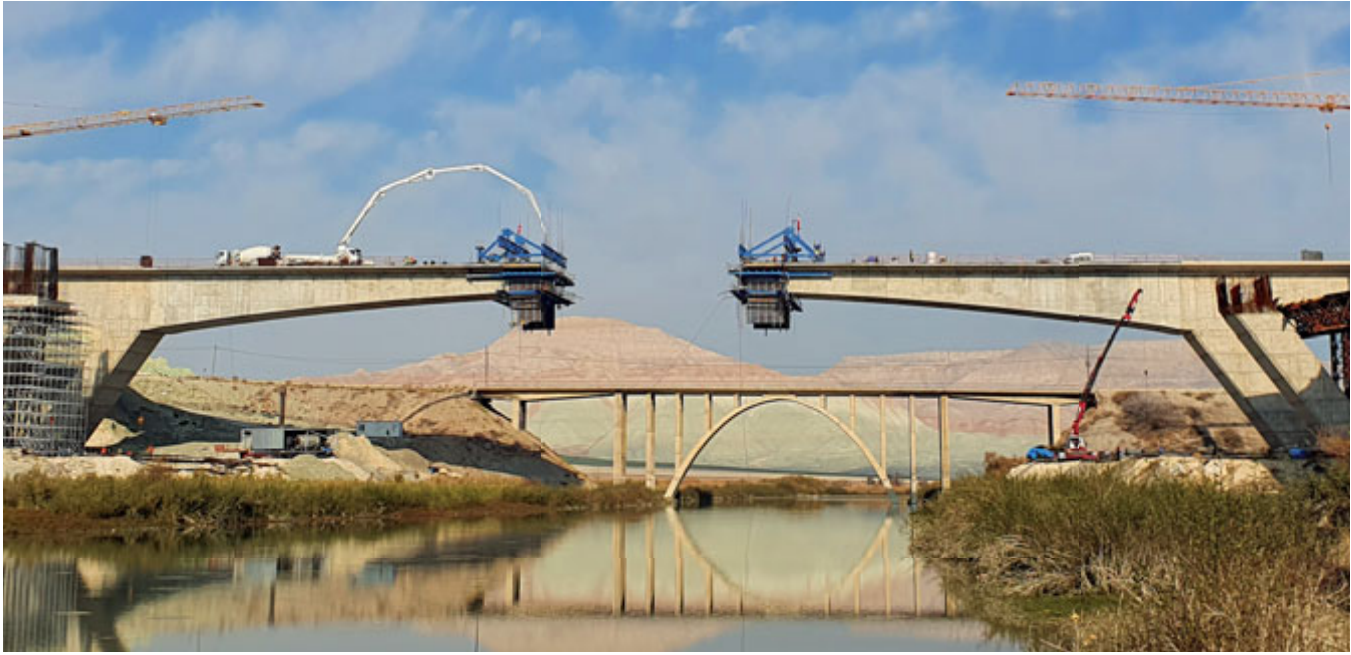
The first of the twin carriageways for the new Çayırhan Bridge – pictured here just before it was completed.
