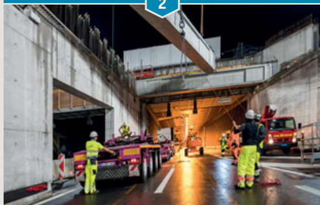
In a carefully planned sequence, each of the 65t beams was delivered to site and lifted into place with the help of a 1,300t crawler crane – the largest in the country.
