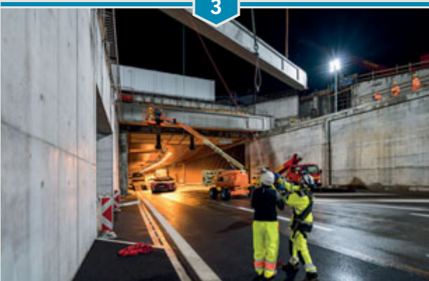
The lifting procedure was repeated for 22 nights until all 186 prestressed beams – and a further 434 roof elements – had been raised and positioned. By the end of the operation, a total weight of 11,700t had been lifted.
