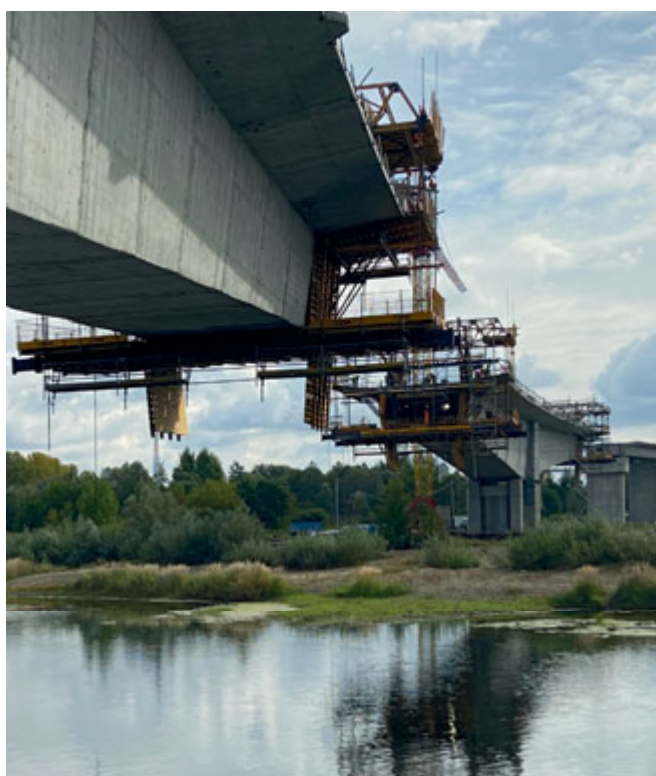
2022 – the new SAG Tarnów Bridge nears span closure and has now overtaken BBR Polska's earlier record for constructing the longest cantilever span in Poland.
