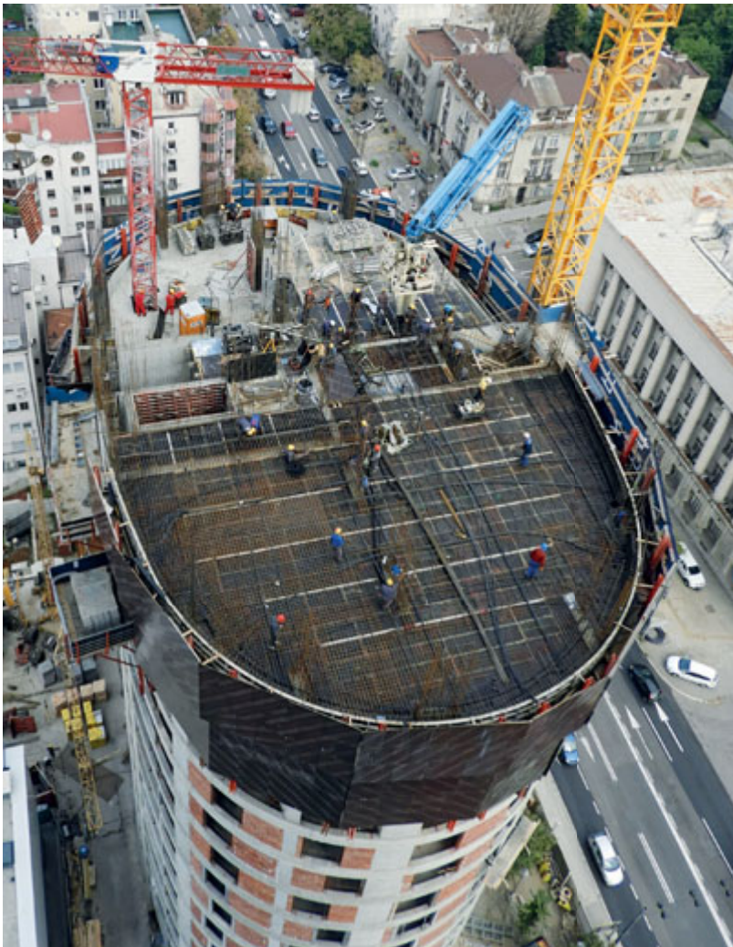
The upper 17 floors of Tower B of the Belgrade Skyline development are elliptical in shape, while the first 10 floors are rectangular. To reduce slab deflection and shear forces, BBR Adria are installing CONA CMM monostrand unbonded PT tendons.
